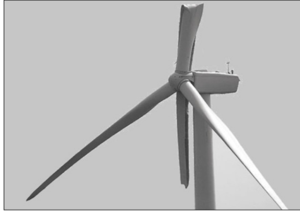
Figure 3: An example of catastrophic blade failure in a wind turbine.
